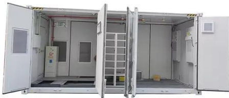
1075KW HH ESS
