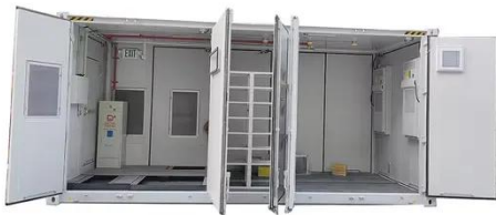
1075KW HH ESS
